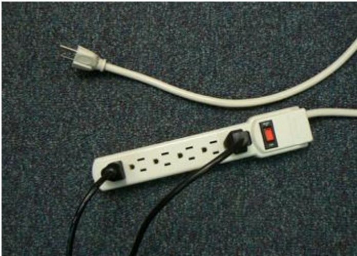
Power Supply Cable Plugged into Power Strip
